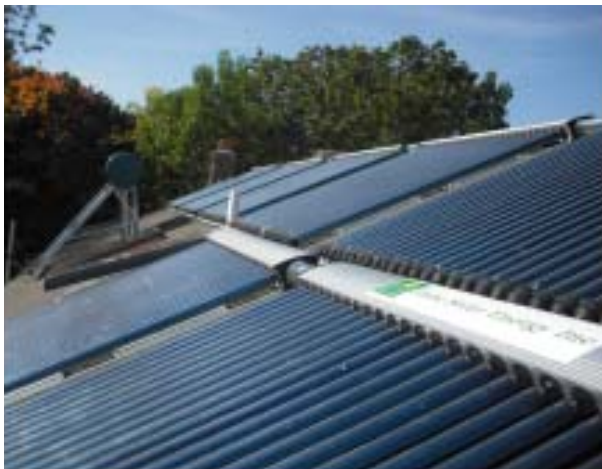
Exhibit 7: Solar Hot Water Panels
