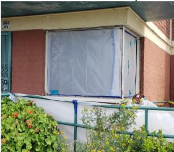
Before: Existing steel windows were cut in several places and pried away from the building's brick structure by an abatement company
