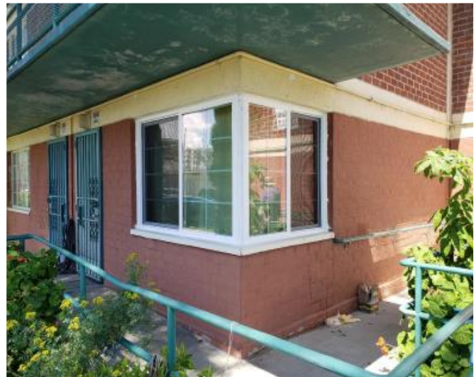
After: New vinyl sliding windows have dual pane glass filled with Argon gas for energy efficiency
