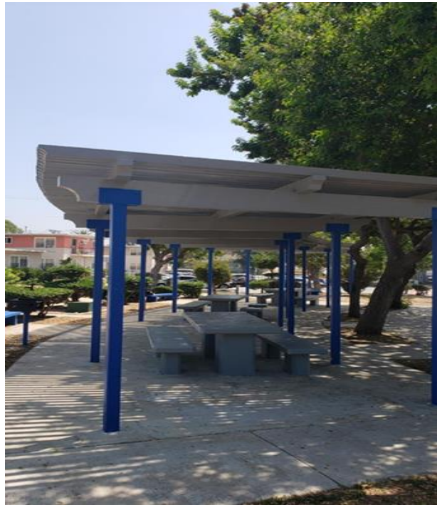
After: The canopy above the patio was replaced. New paint was applied to the canopy as well as the columns
