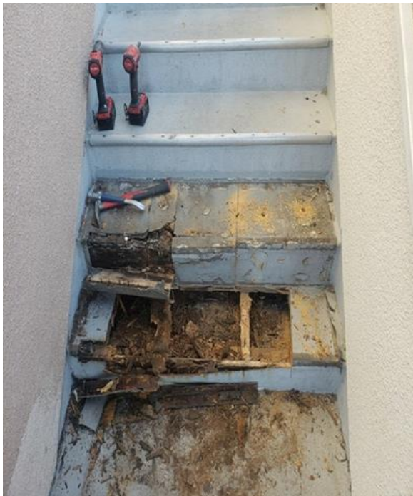
Before: Conditions of the stairs during the initial assessment
