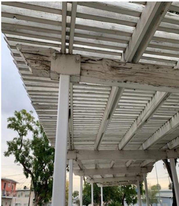
Before: The canopy above the patio had a lot of damage due to age and weather
